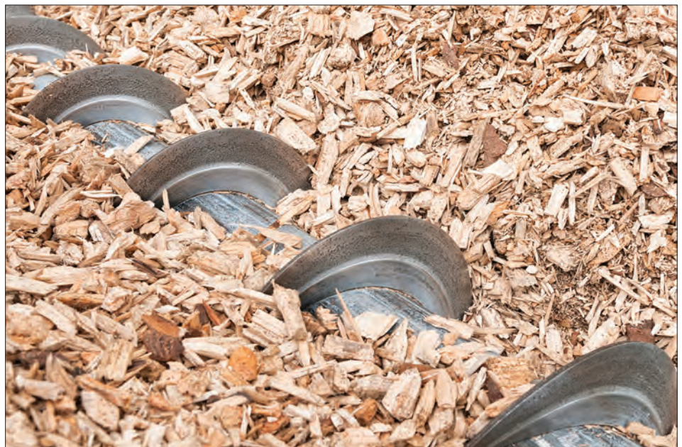
An automated auger loads processed wood chip heating fuel into a biomass boiler.
