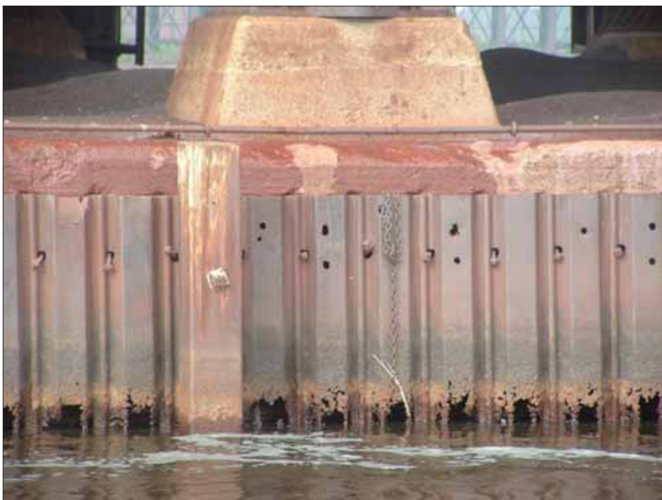
Severe corrosion that has perforated the sheet steel at the DM&IR ore docks near Hallett Dock 5, exposed during low water levels in 2007.
