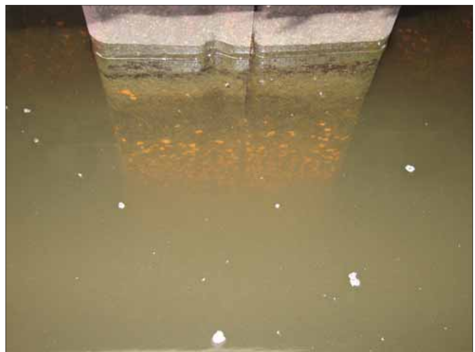
Orange corrosion tubercles below the waterline on a steel piling at the Midwest Energy dock in the Duluth-Superior harbor.
